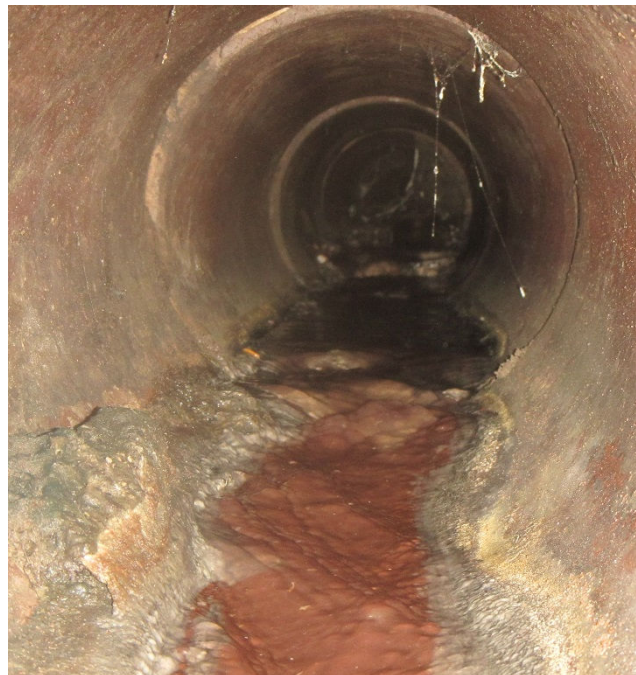
Photo 3-4. Site 7 southwest drop inlet, offset joints
