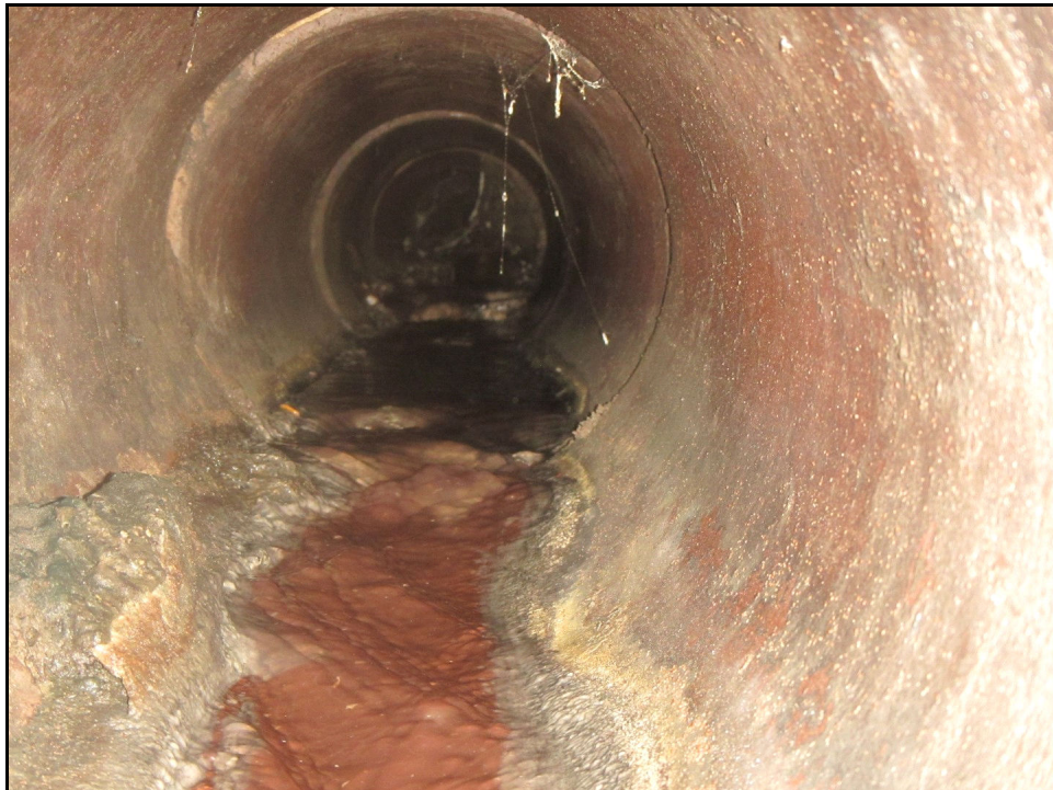
Northwest Influent Pipe
