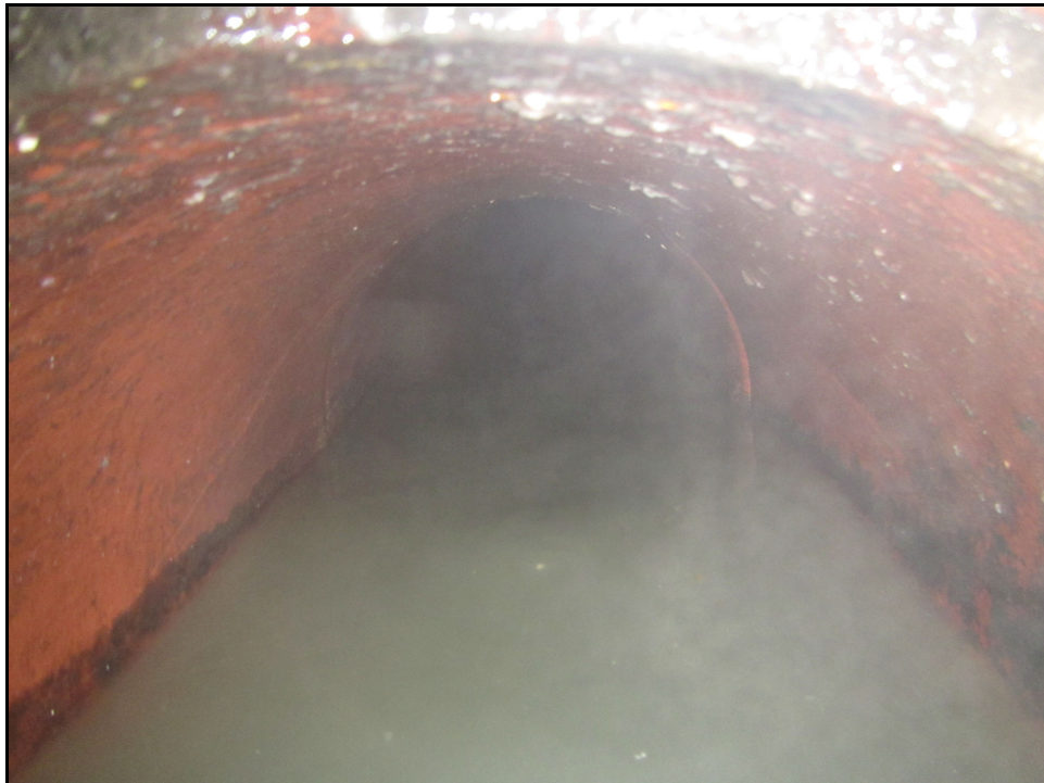
Southwest Influent Pipe
