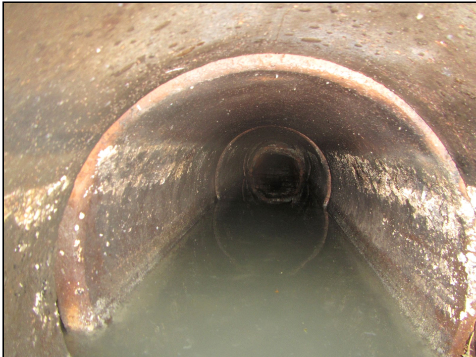
Northwest Influent Pipe
