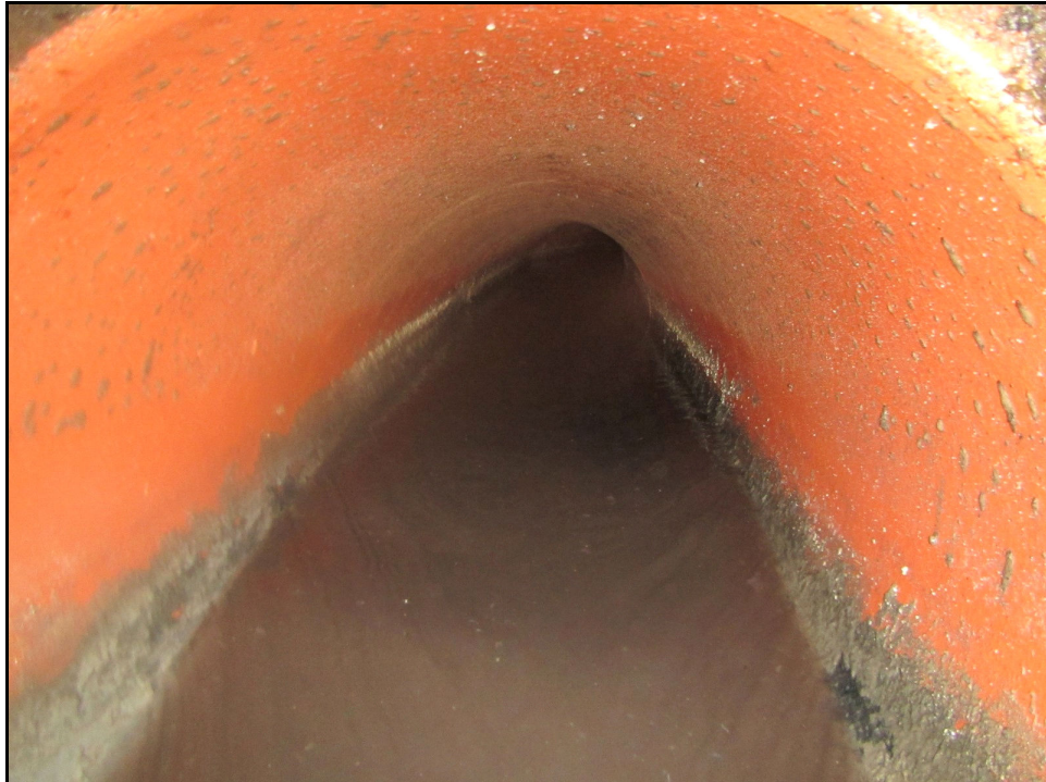
Southwest Influent Pipe
