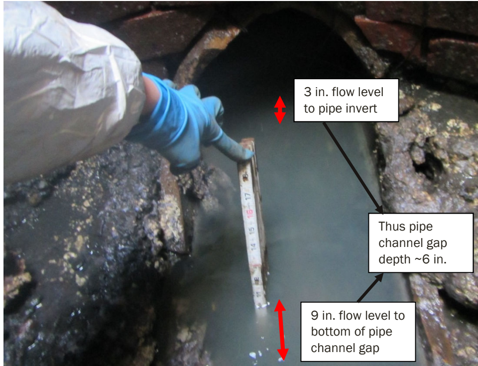
Photo 3-6. Site 9 Pipe Channel Gap
