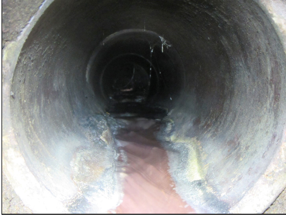
Southwest Influent Pipe
