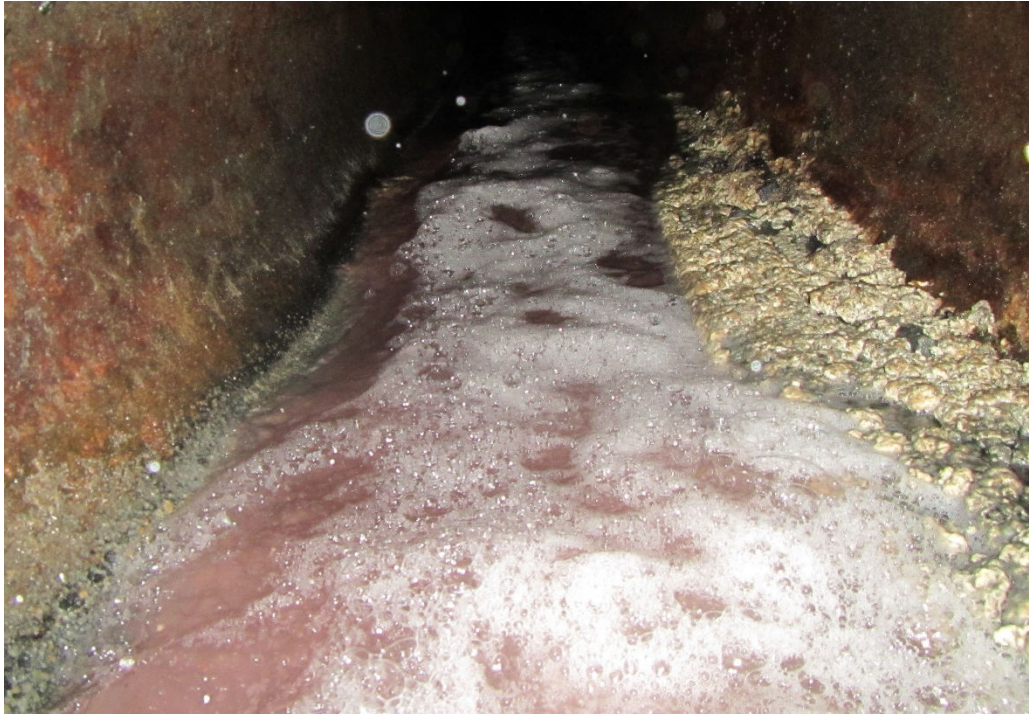
Photo 3-1. Site 4 Southwest Influent Monitored, Pink Flow
