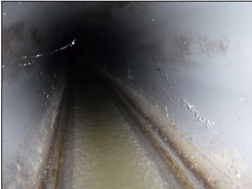
Monitored West Influent Pipe
