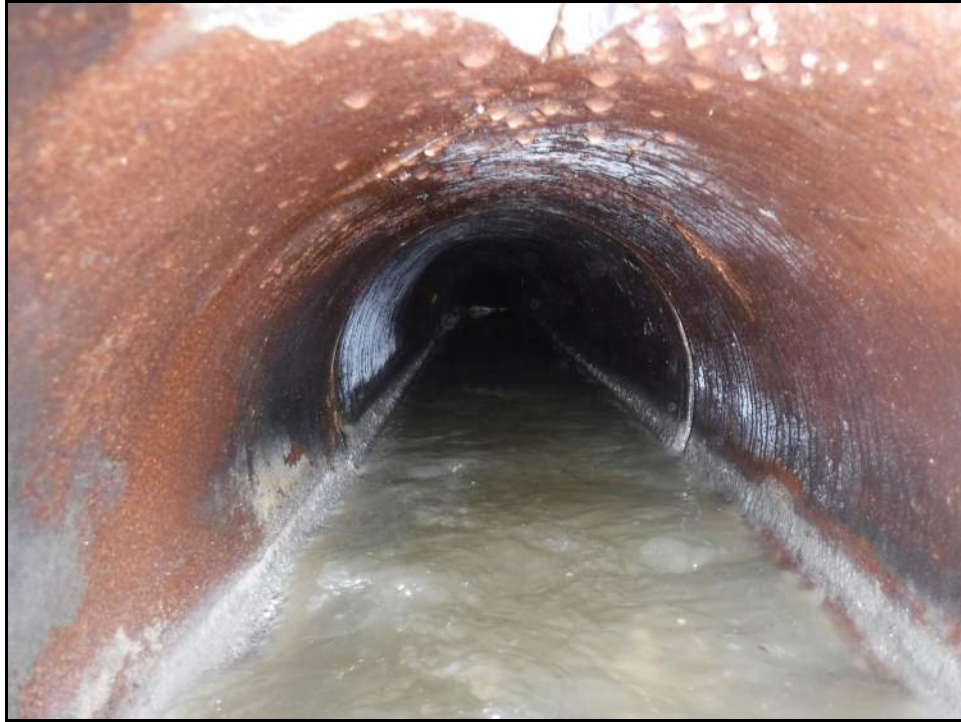
Monitored Effluent Pipe
