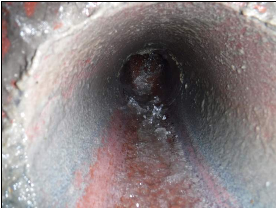
Monitored Lower Influent Pipe
