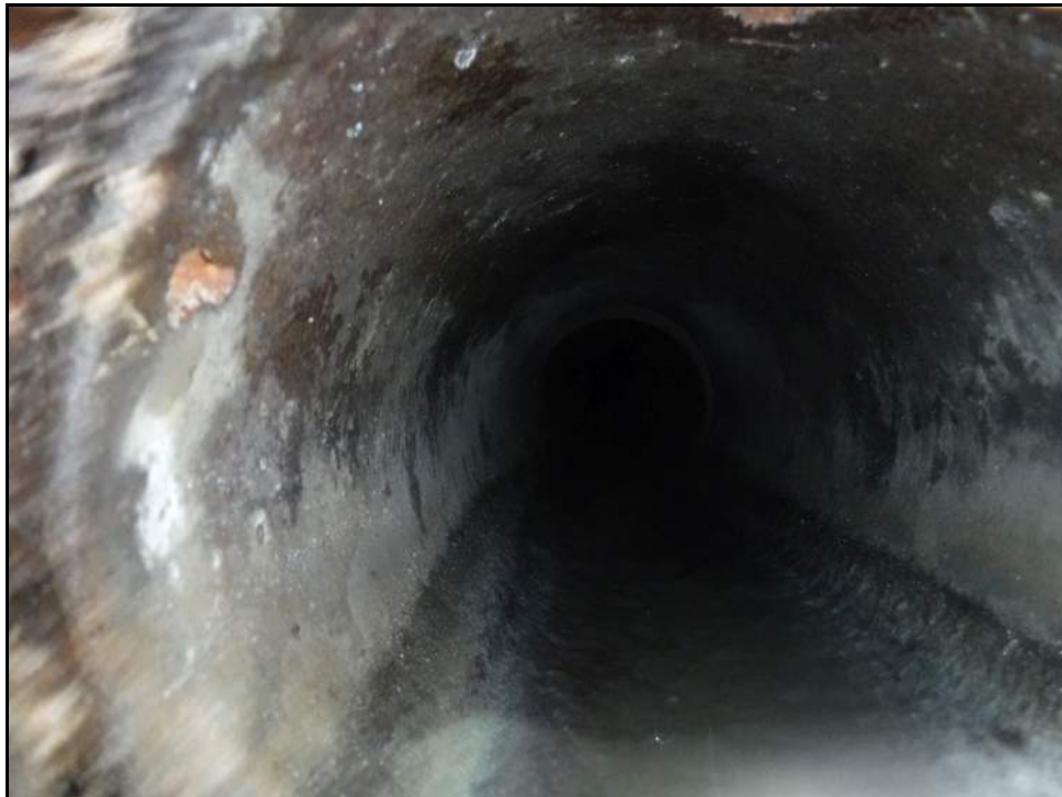
West Influent Pipe
