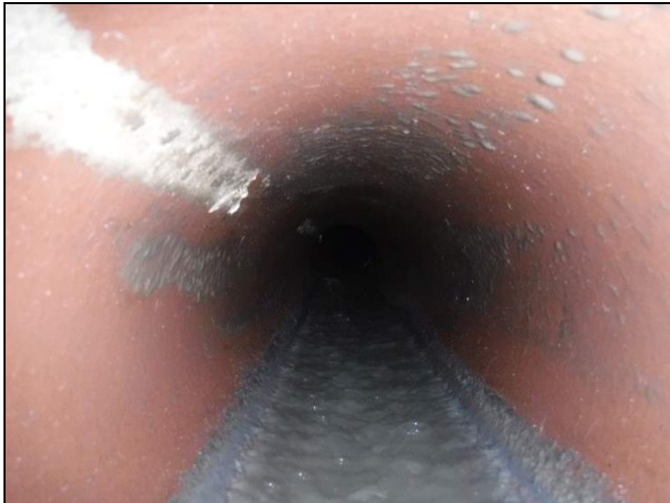
Monitored Northwest Influent Pipe
