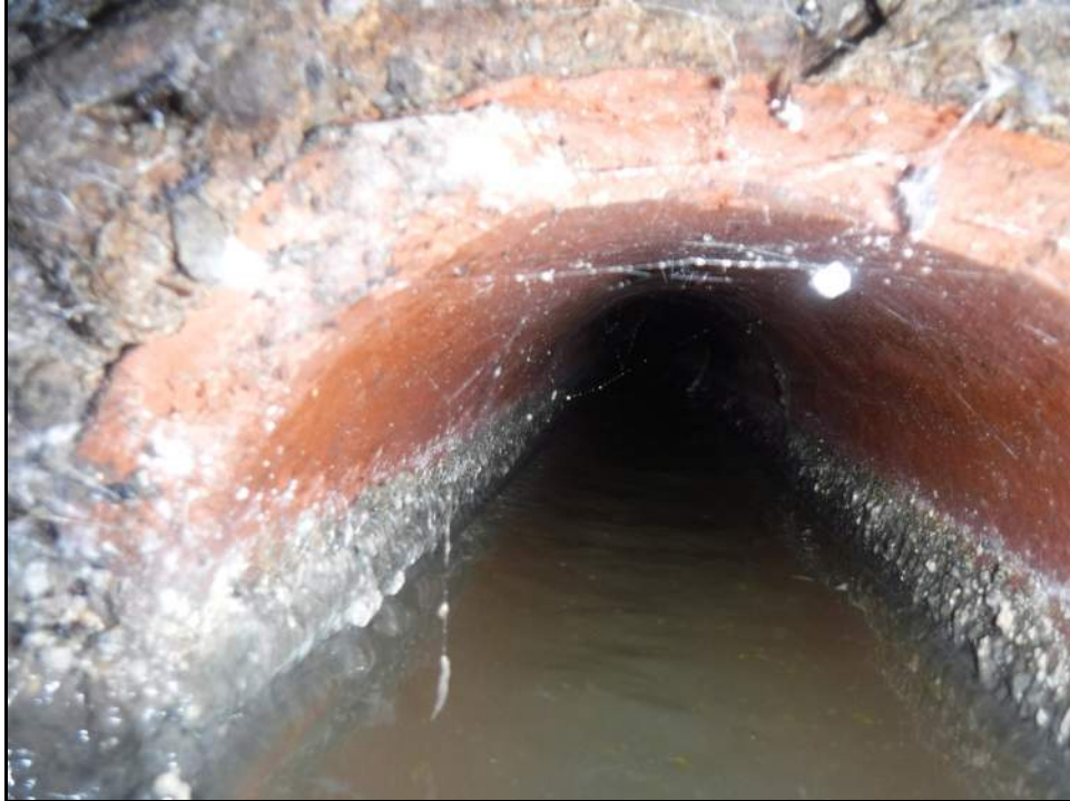
West Influent Pipe
