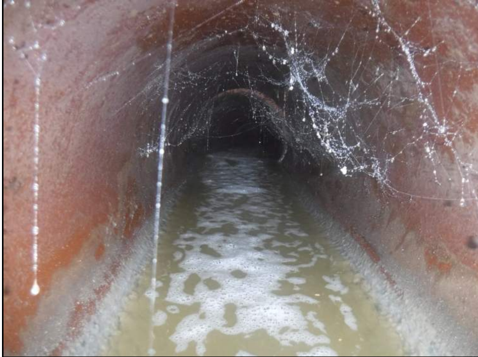
Northwest Influent Pipe
