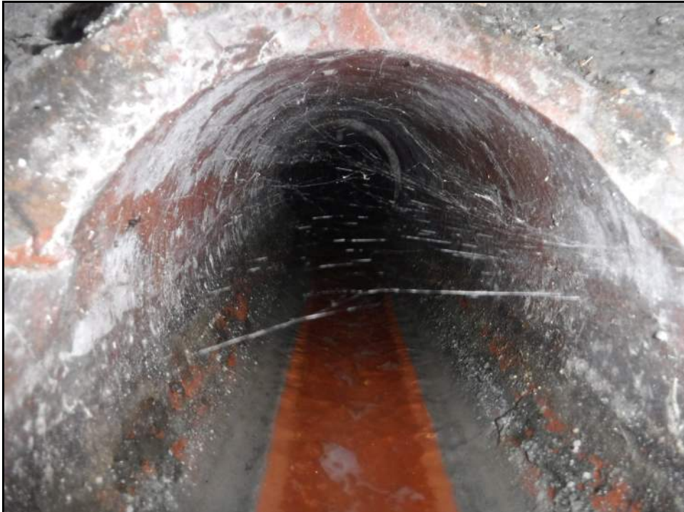
Monitored Influent Pipe
