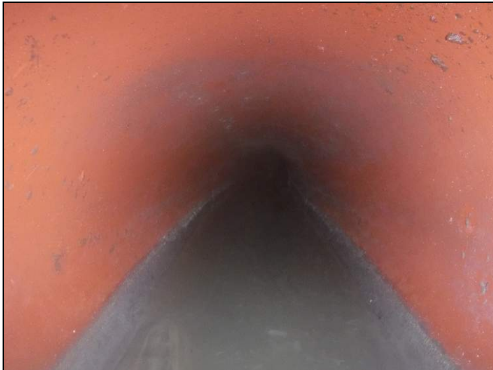
Monitored Northwest Influent Pipe
