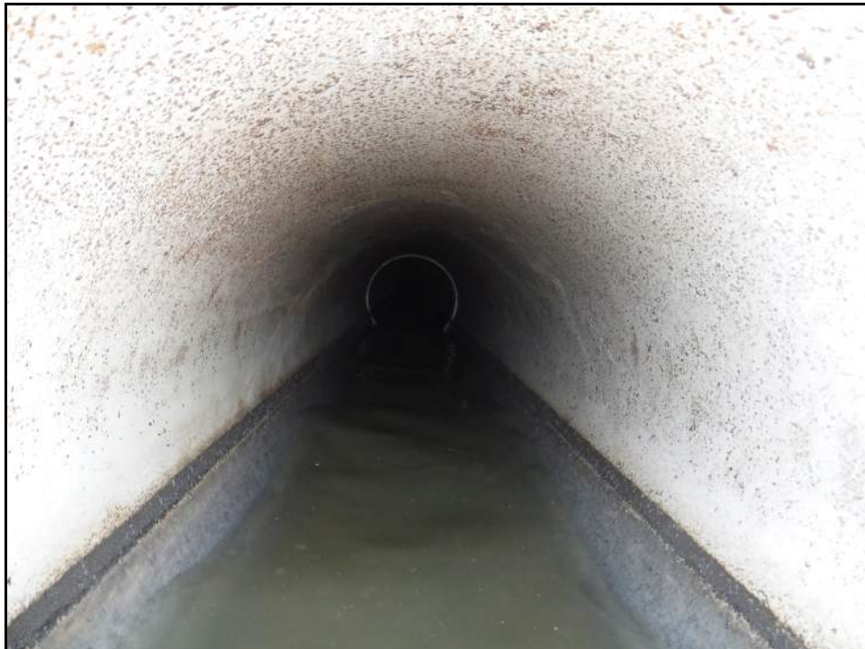
Monitored Influent Pipe
