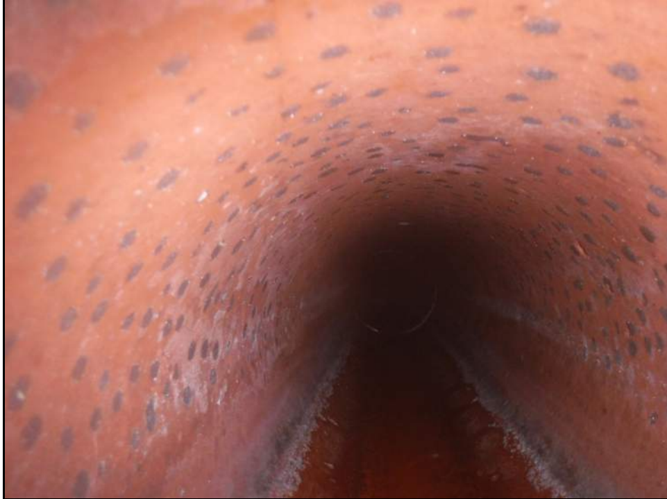
Southwest Influent Pipe
