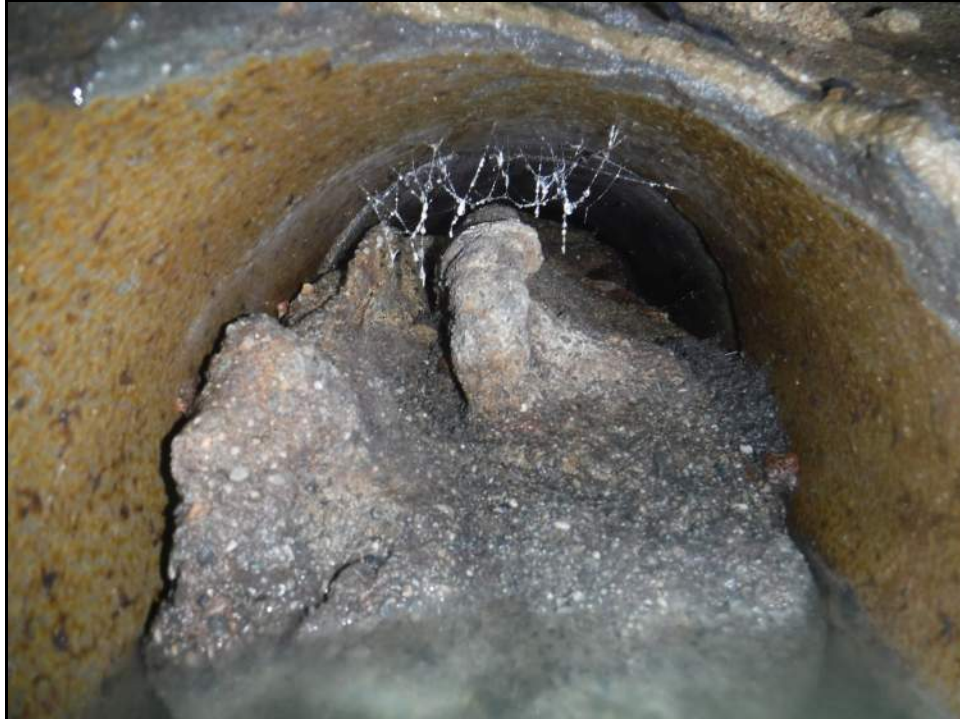
North Influent Pipe
