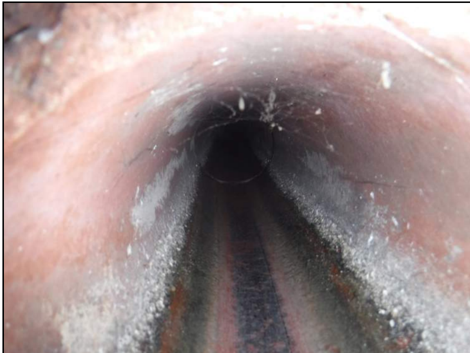
Monitored West Influent Pipe
