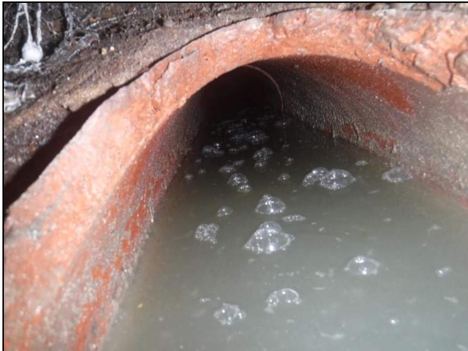
Monitored West Influent Pipe
