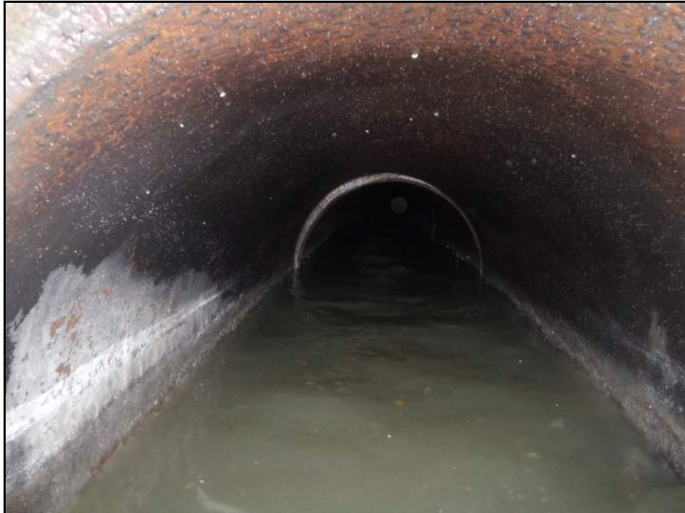
Monitored West Influent Pipe
