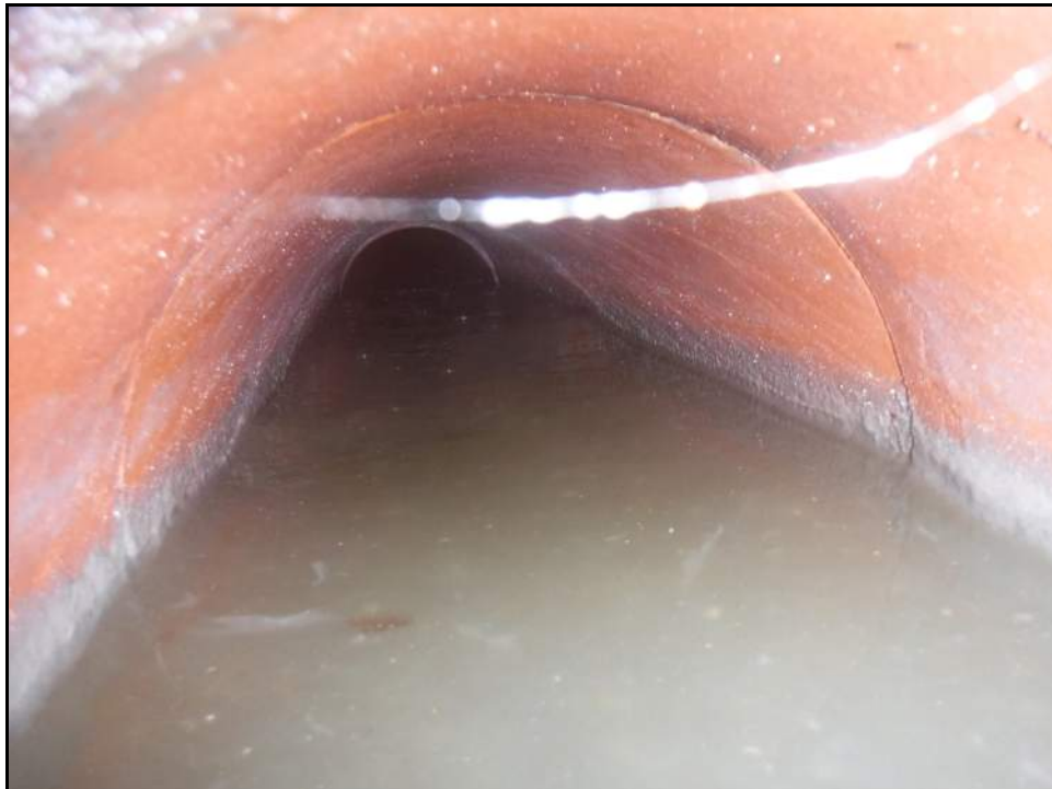
Southwest Monitored Influent Pipe
