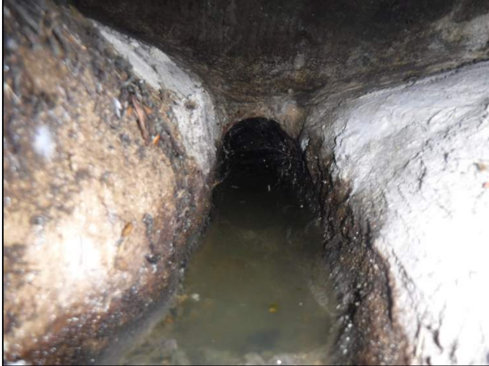
North Influent Pipe
