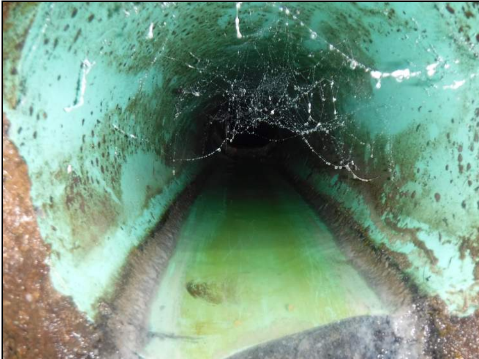
Monitored Northwest Influent Pipe
