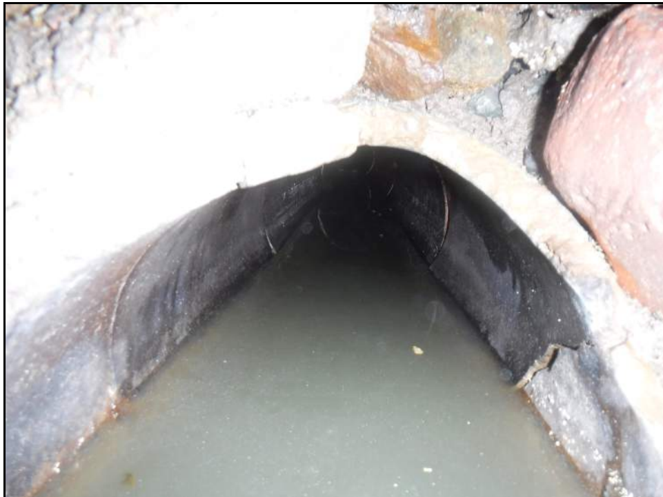
South Influent Pipe
