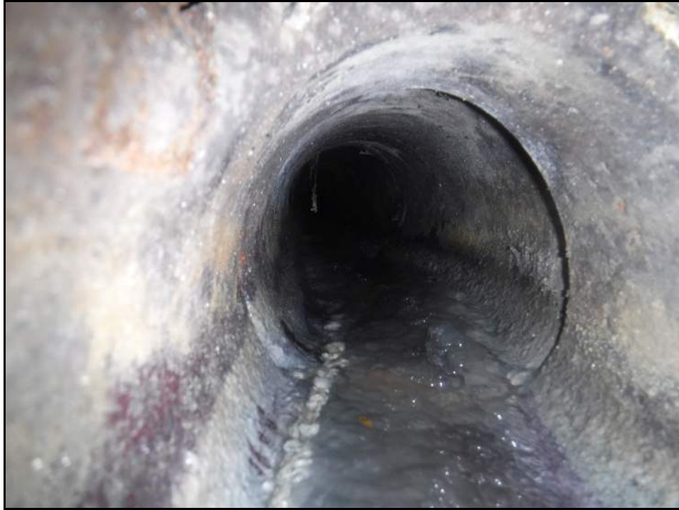
Monitored Effluent Pipe
