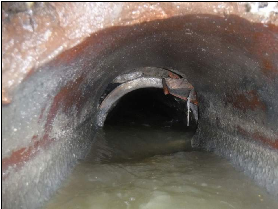
Monitored Influent Pipe
