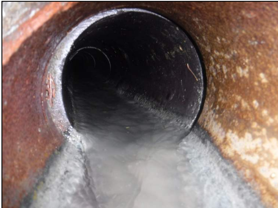
Monitored Northwest Influent Pipe
