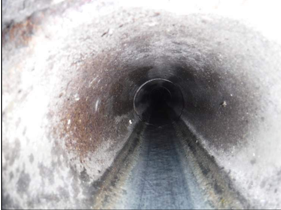
North Influent Pipe
