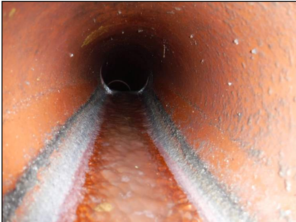
Monitored West Influent Pipe
