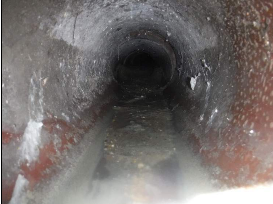
Northeast Influent Pipe
