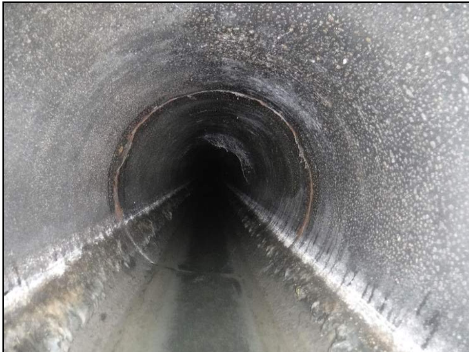
Monitored Influent Pipe
