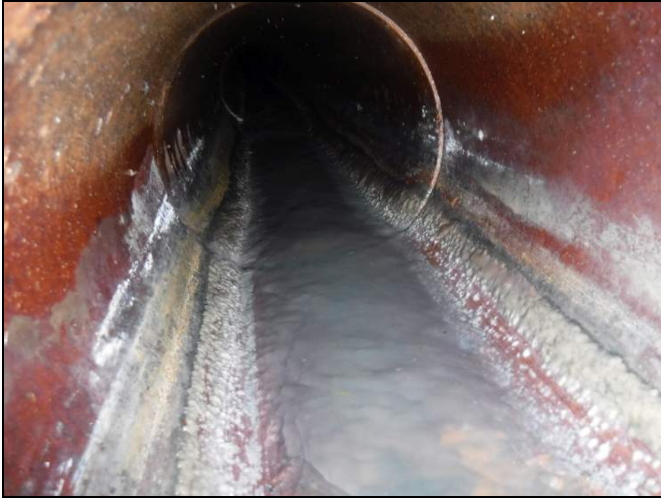
Monitored Effluent Pipe
