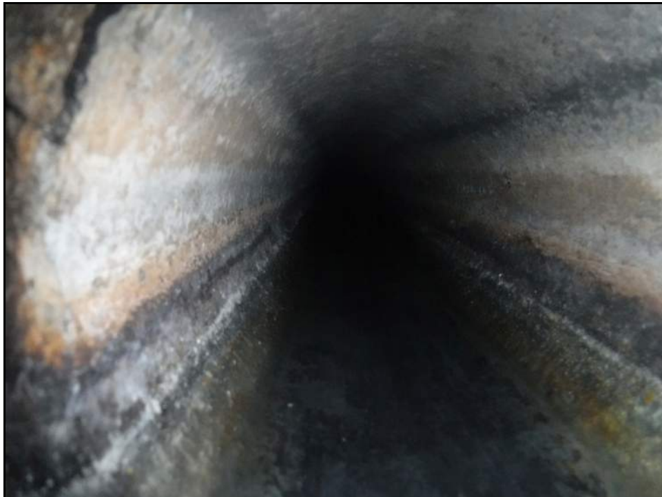
Monitored Influent Pipe
