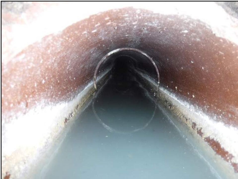
South Influent Pipe
