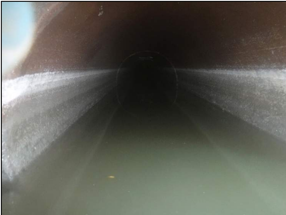
Monitored Southwest Influent Pipe
