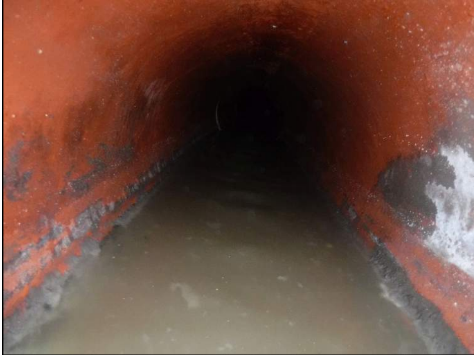
West Influent Pipe
